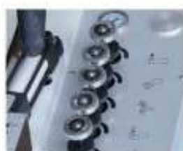
Hydraulic pressure adjustment system
