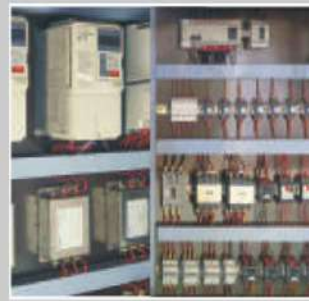
Electrical appliance unit
