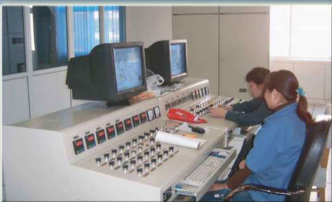
DCS AUTOMATIC Control System
