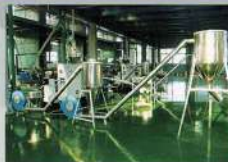
PVC Batching System
