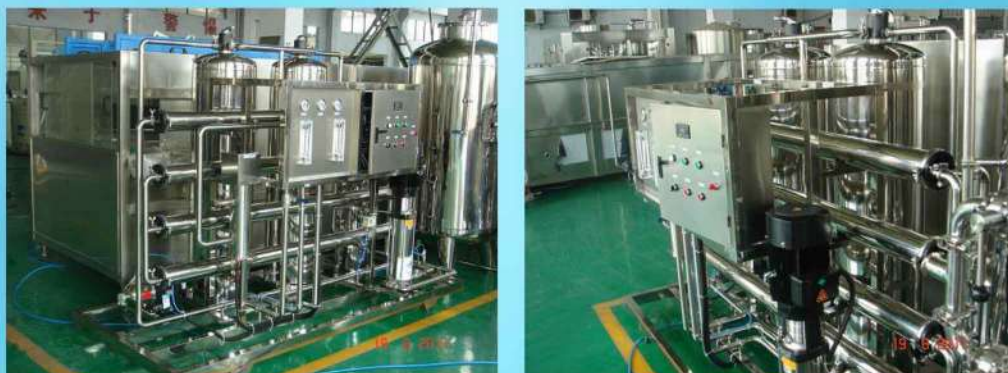
Assembly RO system 1ton/hour No.1-6
