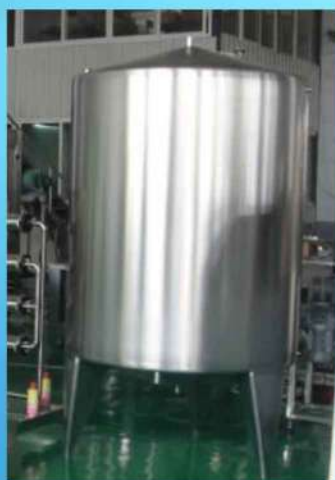
Treated water tank 1 m 3
